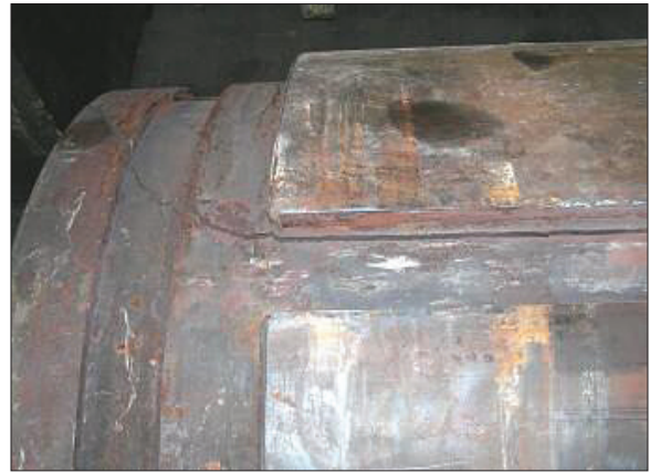
Figure 3. Overheating of container due to aggressive exterior radiation can cause weakening and cracking in the surface of the container as shown here.
